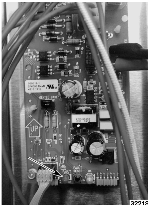
LED FAULT INDICATOR LIGHT ON BOARD
