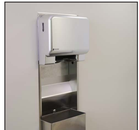
Dispenser is ready to use.
