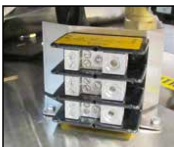
Fig. 3 - Booster terminal block
